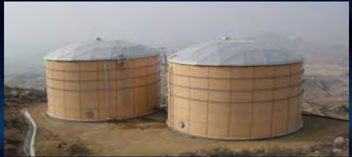
▲ Multiple potable ground storage tank facility.
