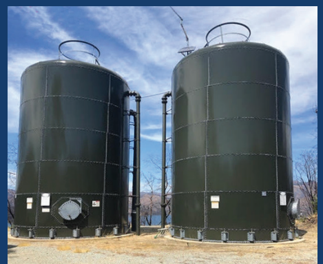
Aquastore tanks looked and performed like new after the Carr Fire came within feet of them.
